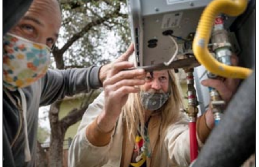
Austin, TX, USA, February 25—Members of the Austin Guerrilla Plumber Corps work to replace a water heater. The corps of five friends worked to repair workers’ plumbing problems caused by the winter storm.
